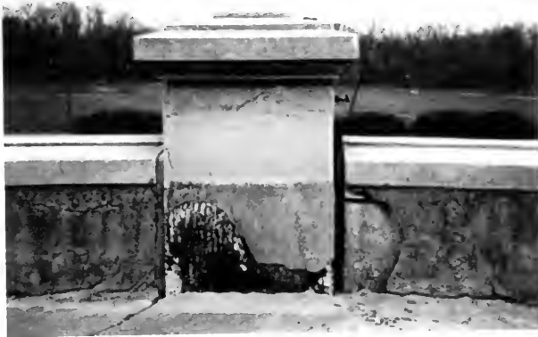
Figure 24: Open joints and mortar loss in the basin wall
